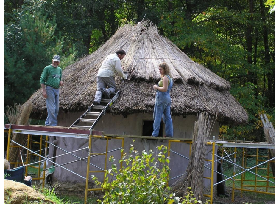
Thatching the cob hermitage: MT Elder--Dan Shuppert, Thatcher--William Cahill, Earthen Finisher—Anna Wolfson.
